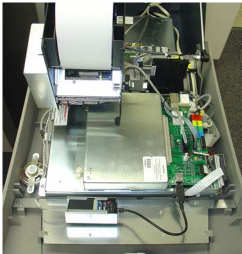
Open control panel.
