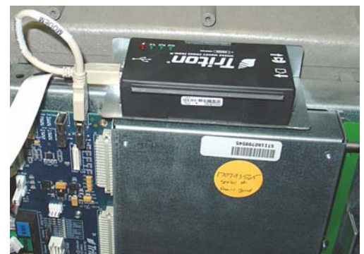
New modem installed/connected.
