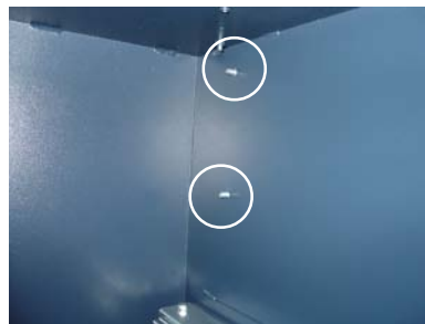
Figure 8. Mounting bolt location.
