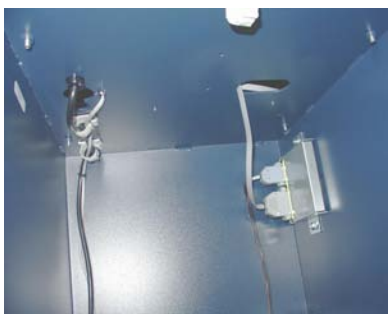
Figure 12. EJ to Docking board cable.
