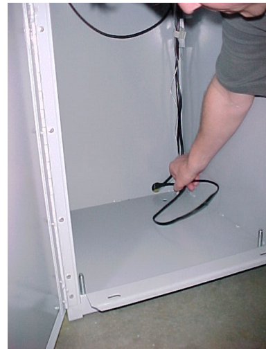
Figure 3. Feed cable out access hole in rear of vault.
